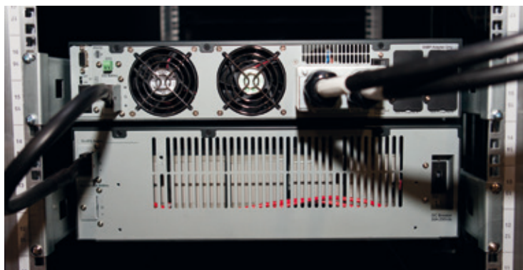
Power distribution rack: UPS systeem
