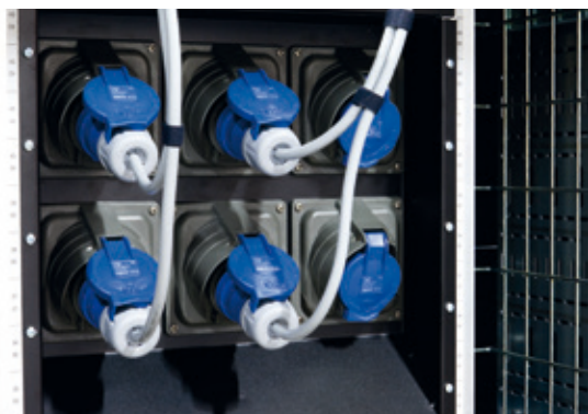
Power distribution rack
